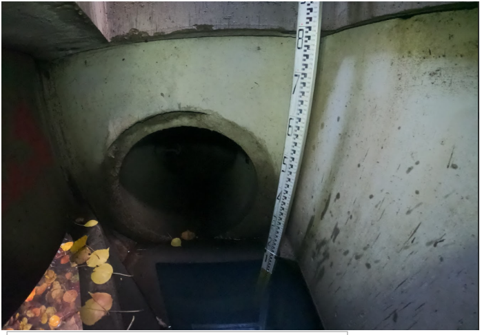
Figure D: Outlet Pipe
